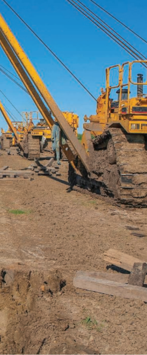
Pipe is laid during construction of a natural gas pipeline in Texas, USA.
